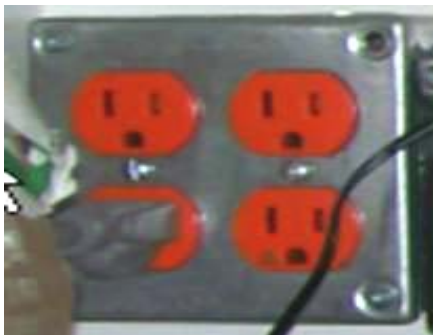
Figure 1 - Double Duplex [4-plex] electrical outlet
